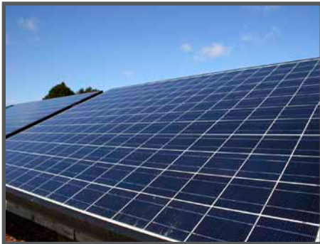
Solar power reduces the County's emissions.
