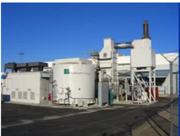
Santa Rita Jail Fuel Cell System
