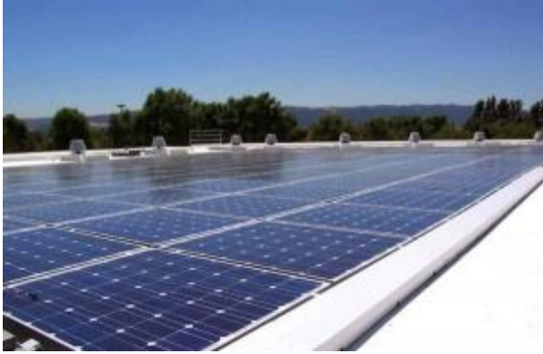
Section of Solar Array Installed at Santa Rita Jail
