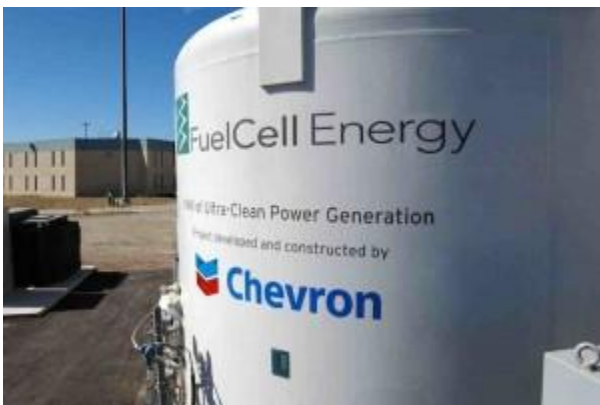
Santa Rita Jail Fuel Cell System
