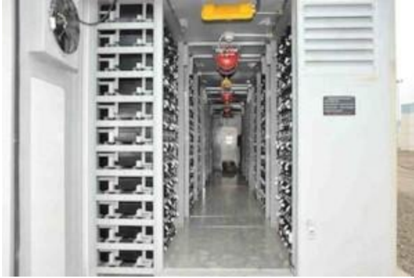
Looking at Battery Storage System Within Storage Container
