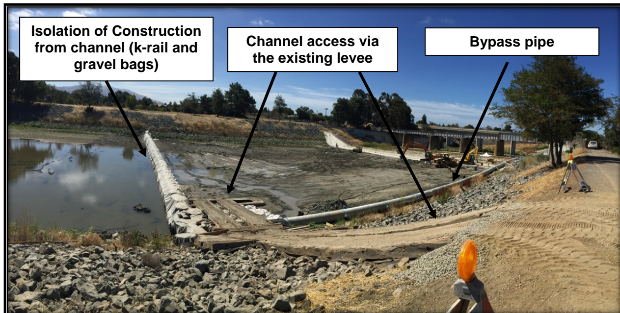
Figure 12. Typical site isolation and construction zones (per the previous ACWD replacement of Rubber Dam 1 fabric).
