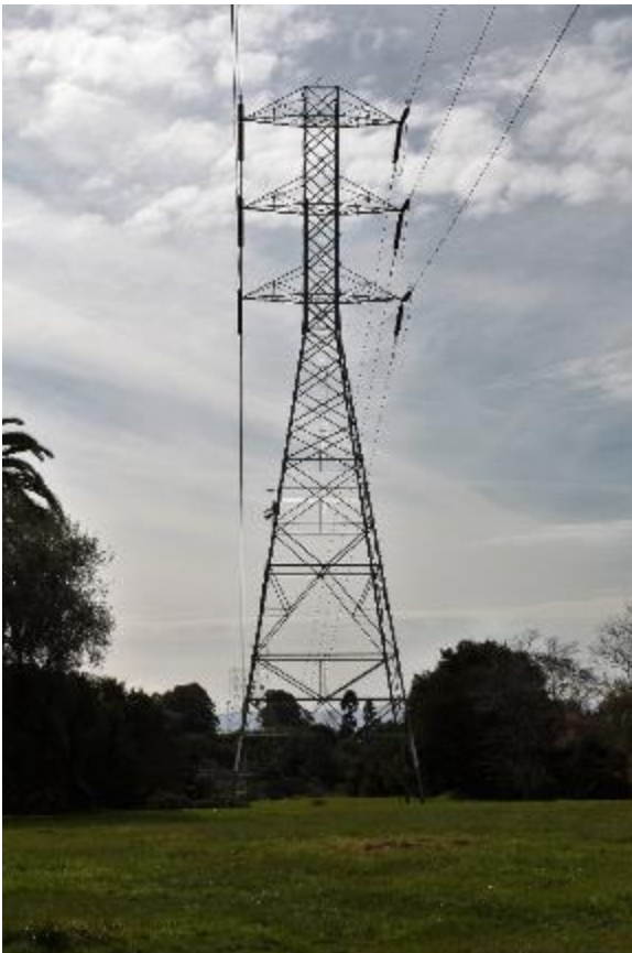
PG&E transmission lines near Second Street
