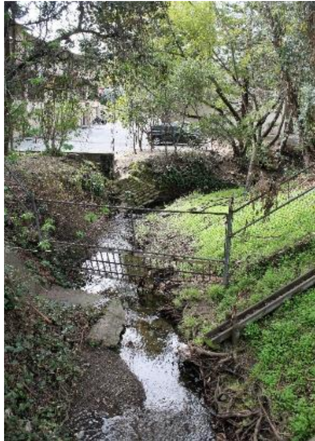
Eroded bank conditions along Sulphur Creek
