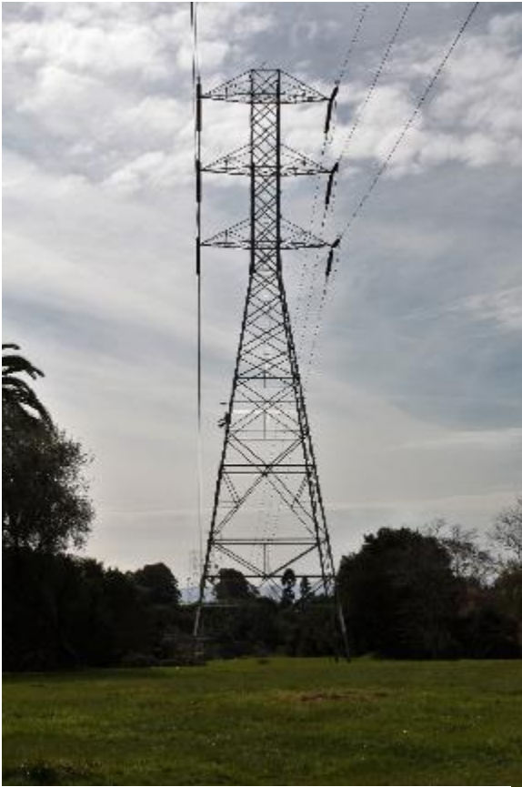
PG&E transmission lines near Second Street
