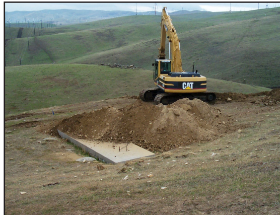
Dirt is moved from the lower bank to fill in the turbine pad area and foundation
