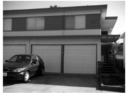
Older “soft-story” buildings with habitable space above garages are some of the more vulnerable building types in the event of an earthquake.
